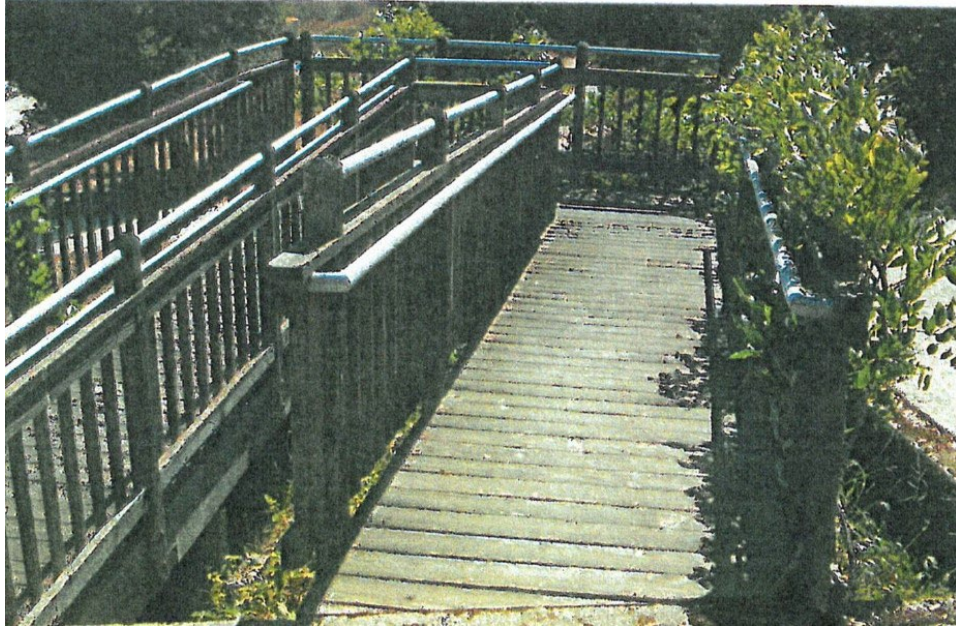
GRRP Ranger Station Wheelchair Ramp to be Replaced
