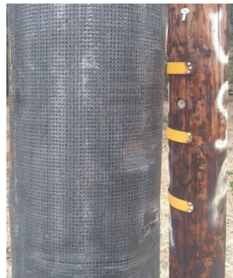
New fire-retardant pole
