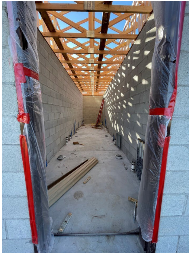
Restroom Building Storage Room Interior Utilities Chase
