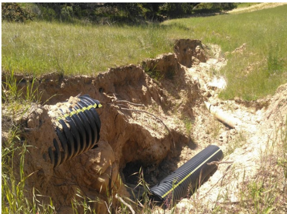
Collapsed and Undermined culvert
