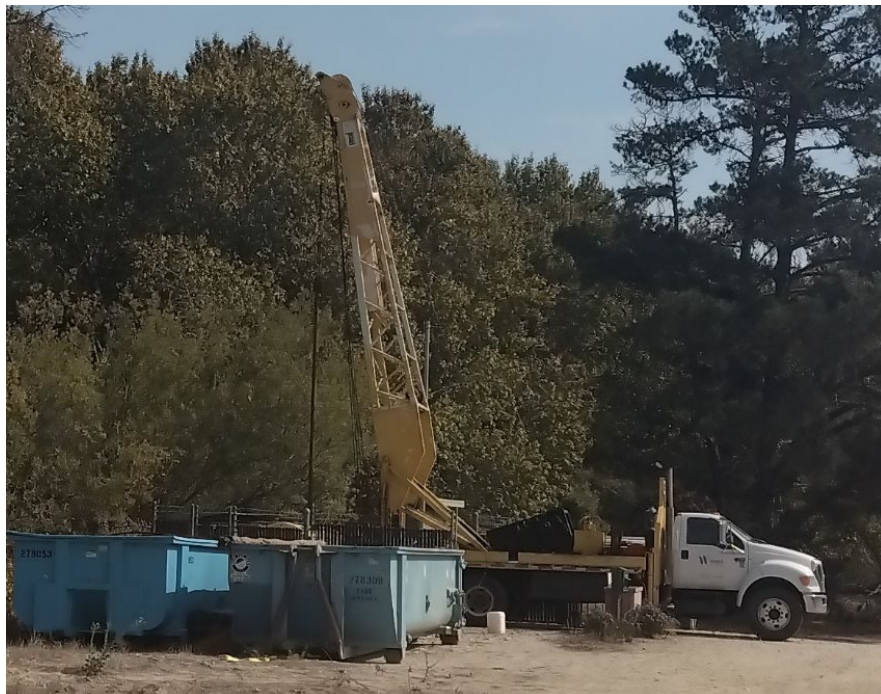
Cal-Am Equipment at Lupine Loop Production Well Site
