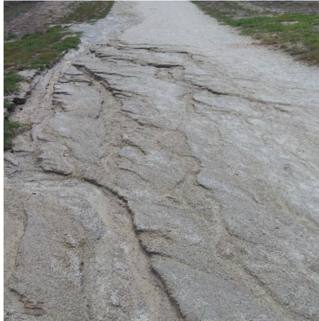
Damage Caused by Recent Rainfall
