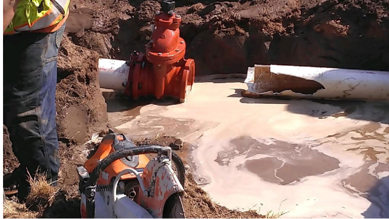
Broken 8” water main owned by MPRPD was repaired
