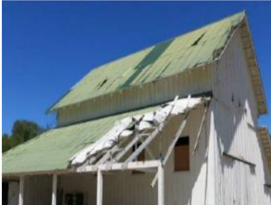
PCRPN Barn Roof Damage
