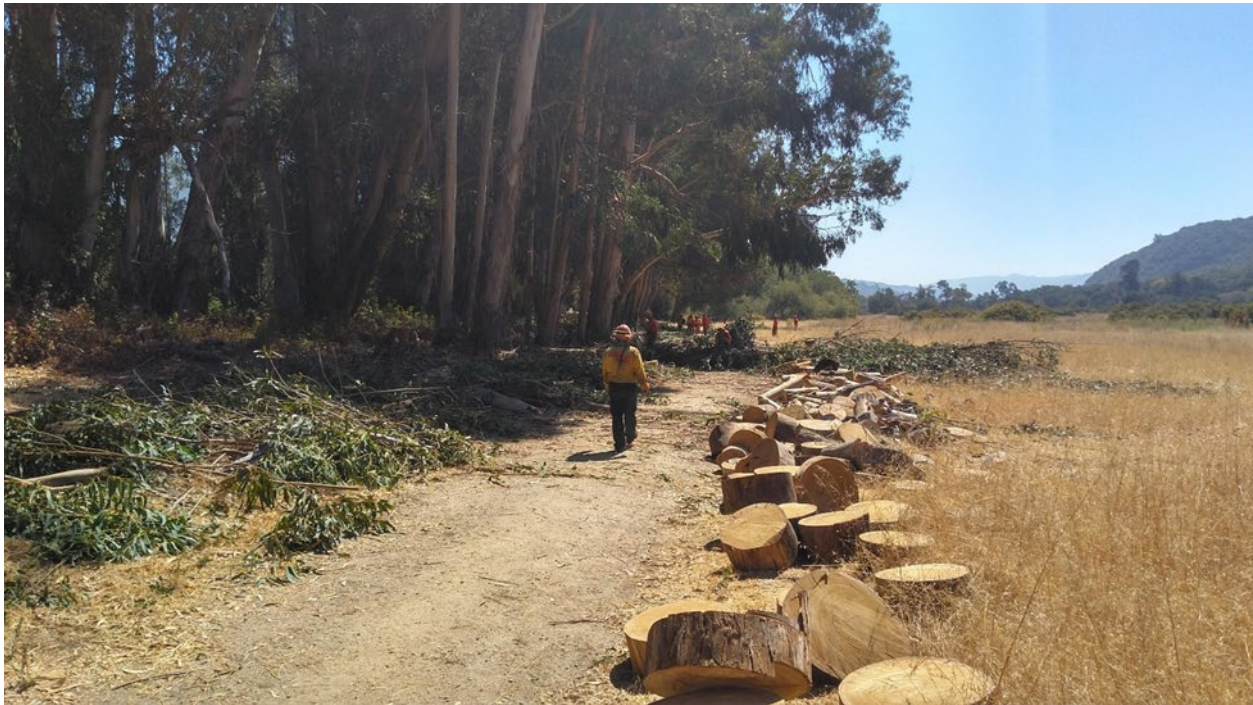
Brush to be chipped (on left) and wood rounds to be relocated (on right)
