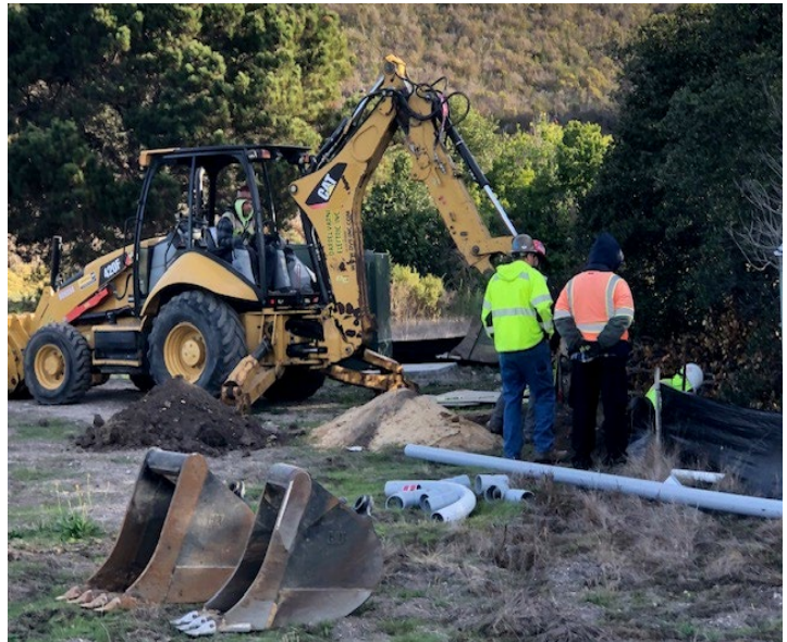
PG&E electrical installation
