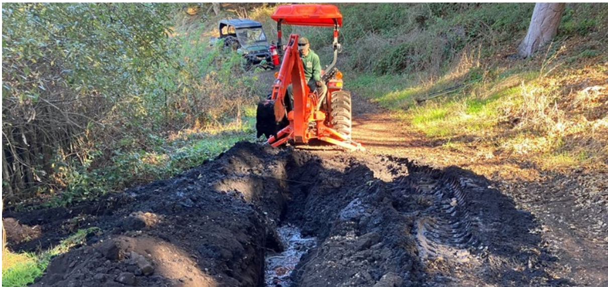
Rangers exposing broken waterline w/ MPRPD equipment
