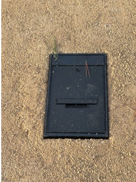
MP Pad electrical box
