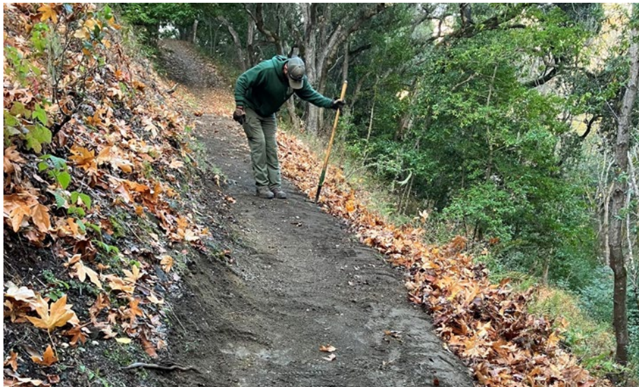
Segment of Live Oak Trail was out-sloped
