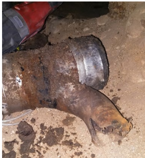
Corroded cast-iron fitting under MPRPD's HQ
