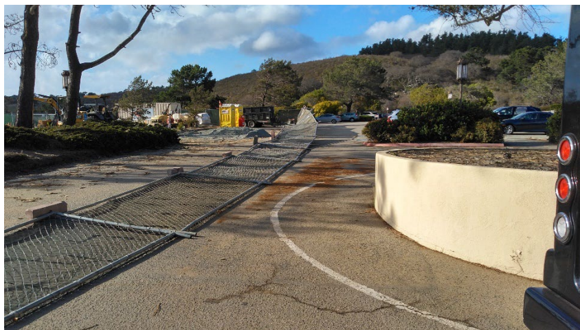
Project-B construction fence blown over by wind
