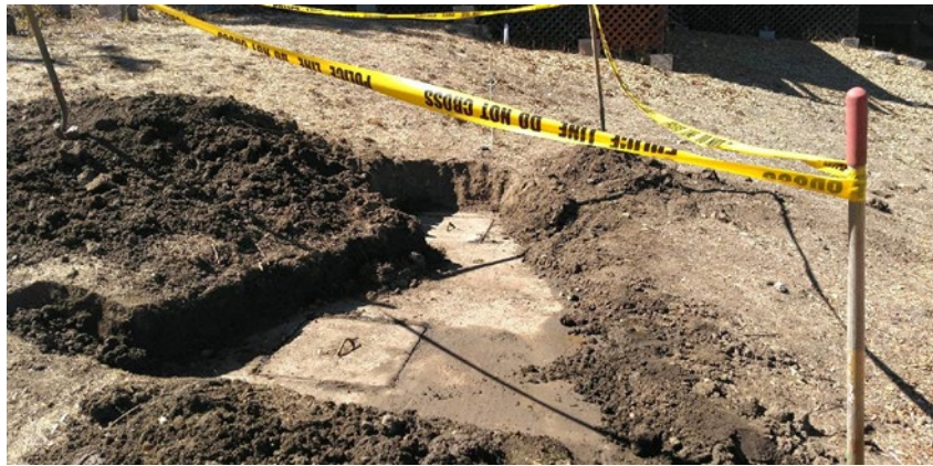
GRRP Ranger Station septic tank lids exposed
