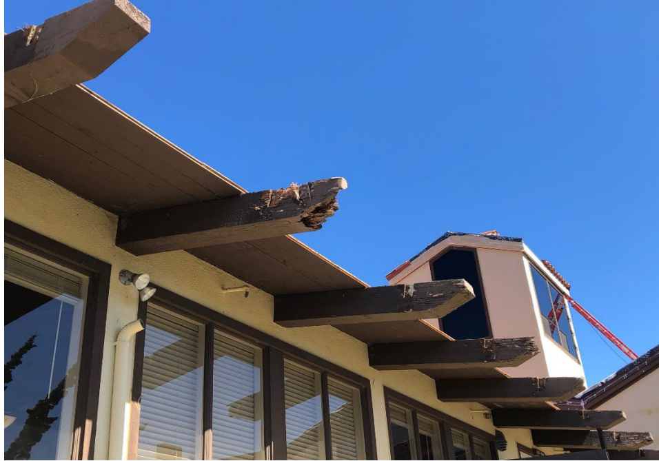
Back side of the Discovery Center (Rotted outriggers to be cut and treated)
