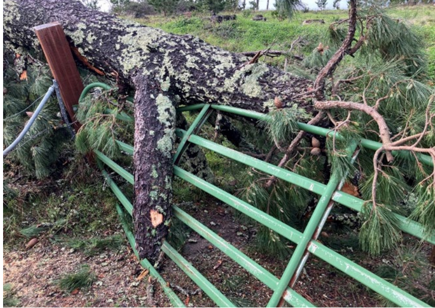
PCRP - Corona Road Entrance Gate Damaged
