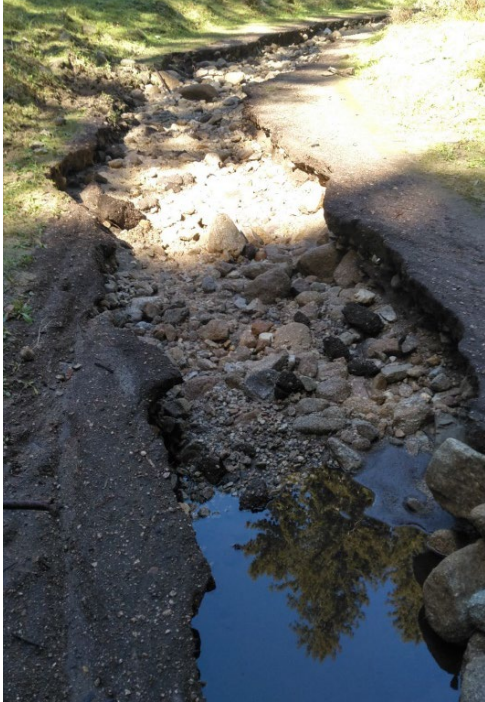
Road damage along PC Trail
