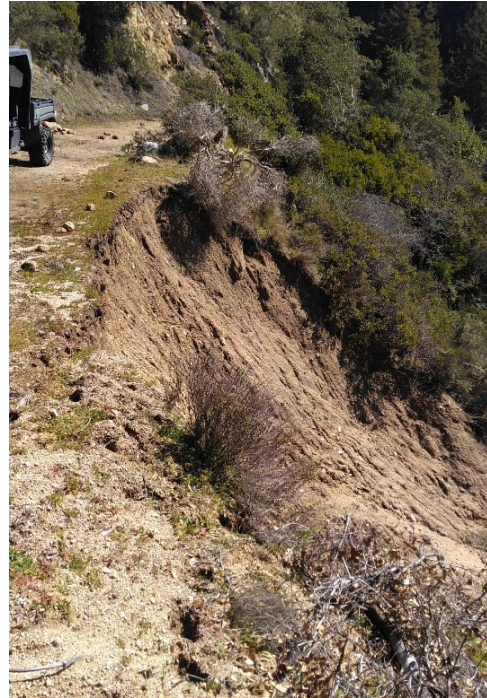
Undermined road in PCRP Backcountry
