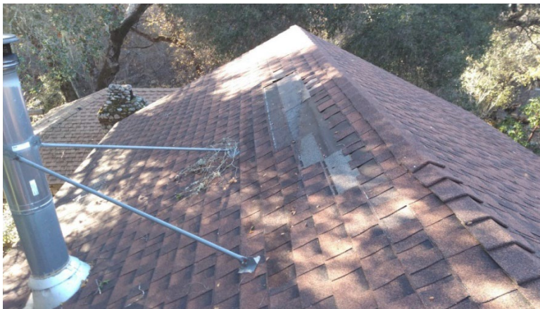
CCC Apartment Roof Damage
