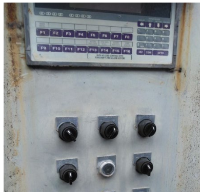
Existing RCU Irrigation Panel
