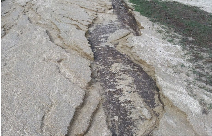
Damage caused by recent rainfall
