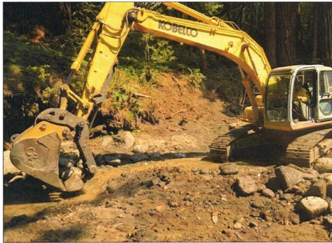
San Jose Creek Crossing repair after Soberanes Fire on August 22, 2016 (Photo by: Christy Wyckoff)
