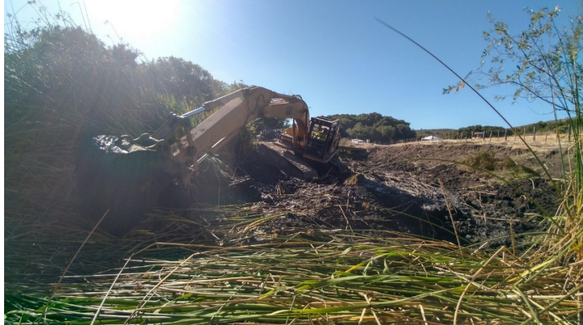
Tom “Little Bear” Nason using his excavator to remove overgrown vegetation and accumulated sediment from Animas Pond
