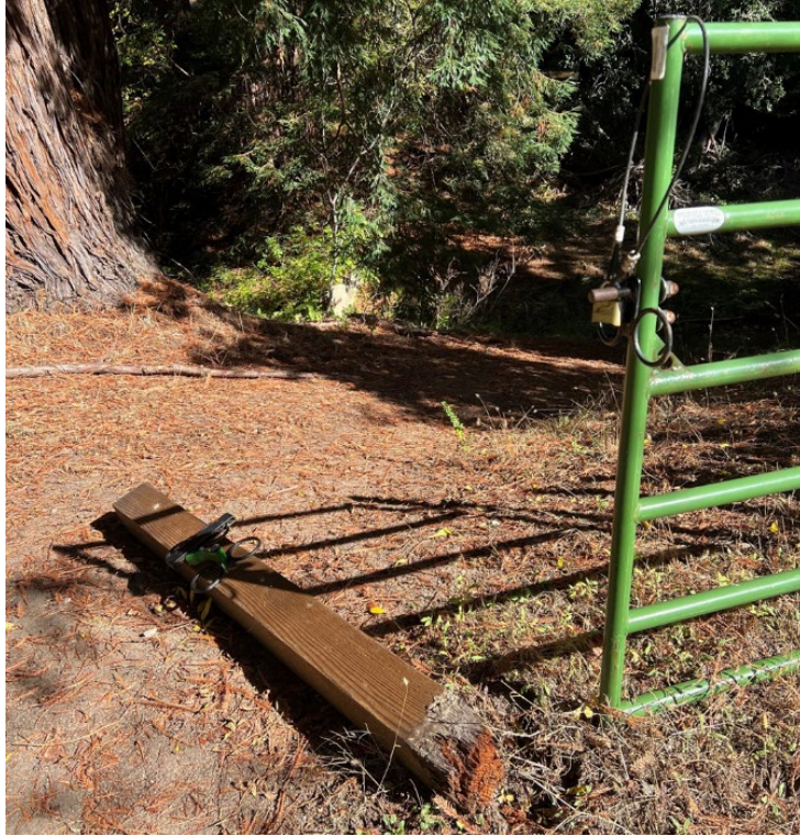
Broken gate post in PCRP Backcountry
