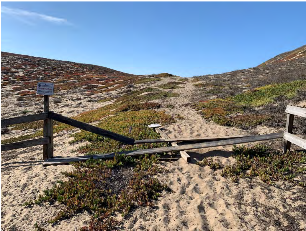
Figure D-4. Trail Closure signs and compromised fence west of sign in Figure C-3.
